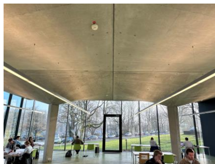
Interior of a pavilion at the RWTH Aachen University of Technology, Germany. The roof structure has been reinforced with carbon fibre textile and is only six centimetres thick. Photographer: RWTH Aachen | Thorsten Karbach
